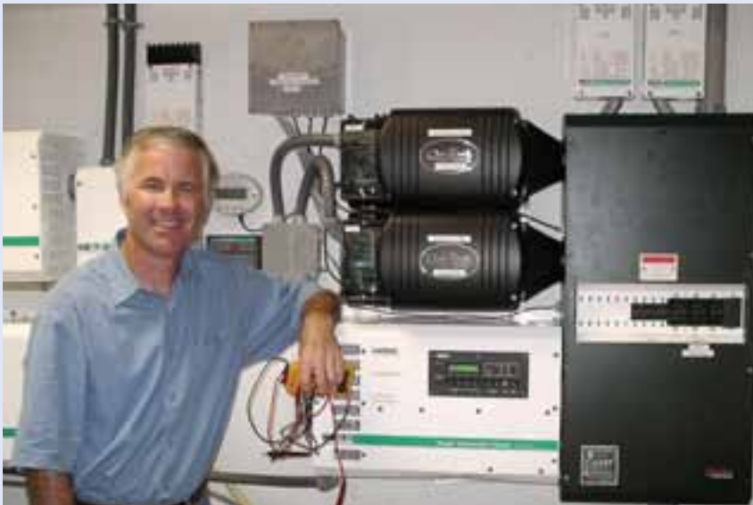
Author and system installer John McNicholas with the first stacked Xantrex/OutBack inverter system made possible by the MIG2 migration board.
